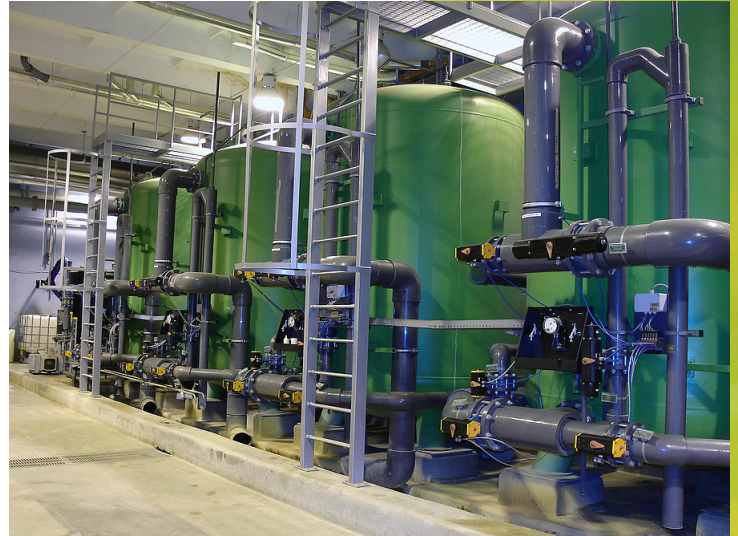
Water treatment plants make water safe to drink.
